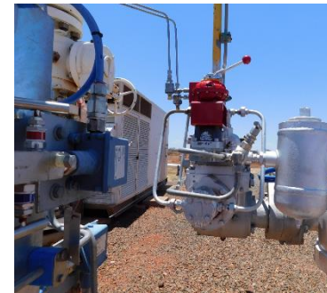
Application with Easytork actuators (in red) driven by natural gas
